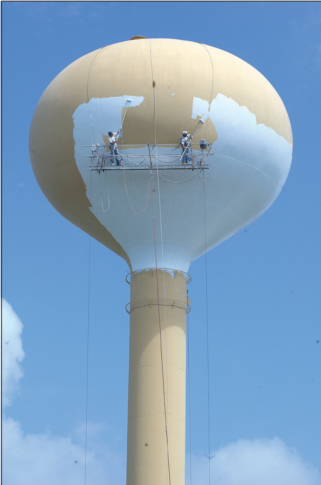
THESE PAINTERS have a bird's eye view of McGregor from their position on McGregor's water tower at Johnson Drive. Repairs to the inside of McGregor's primary water tower are just about completed and awaiting inspection. The outside painting will finish up the project. A City of McGregor logo was added to the structure.
